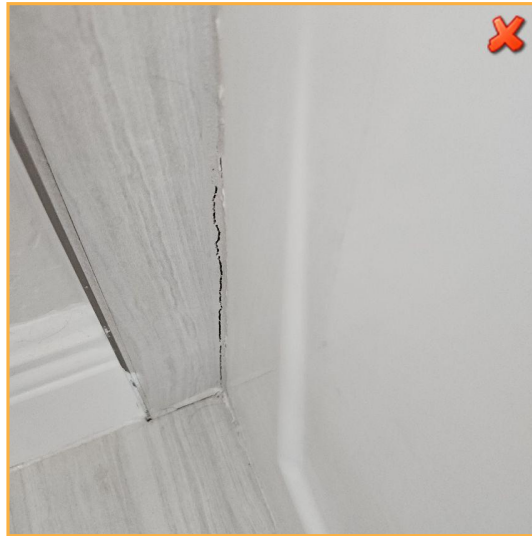
Cracked grout by guest bath tub
