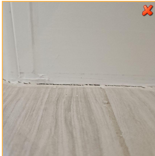
Gaps visible below baseboard
