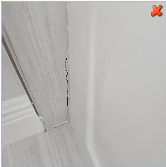
Cracked grout by guest bath tub
