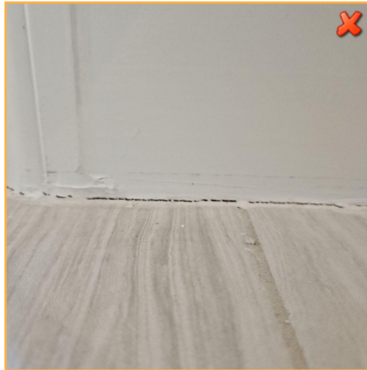
Gaps visible below baseboard
