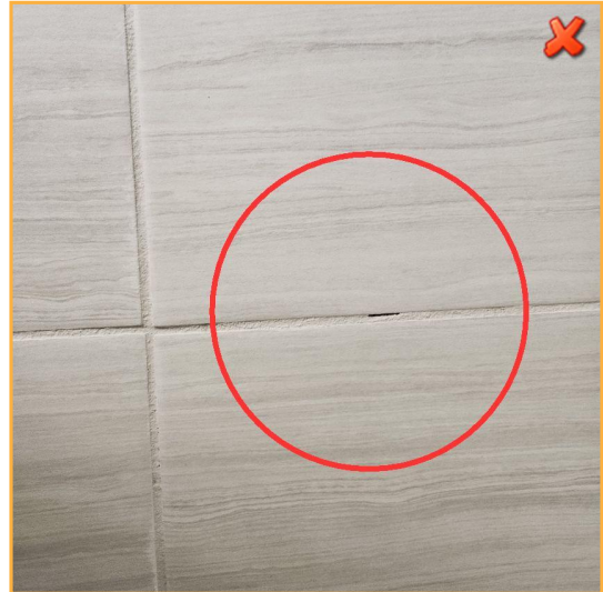
Primary bath shower has areas of missing grout
