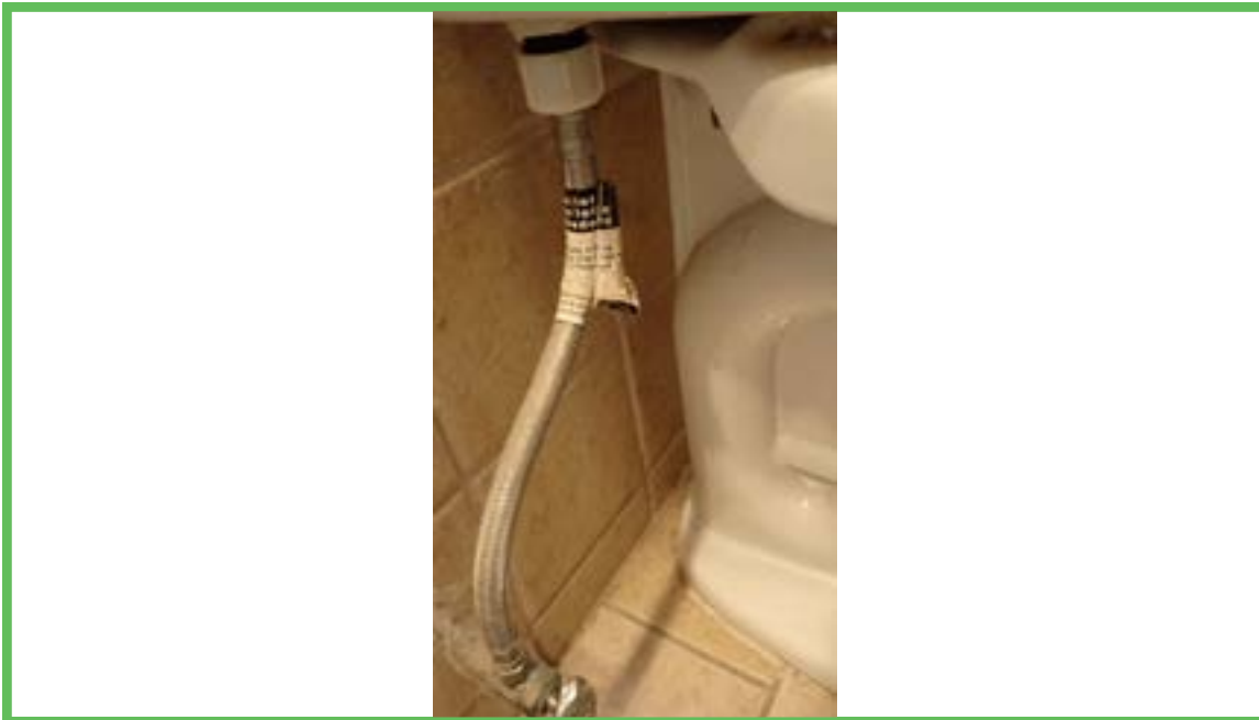
Bath 1 Toilet Valve
