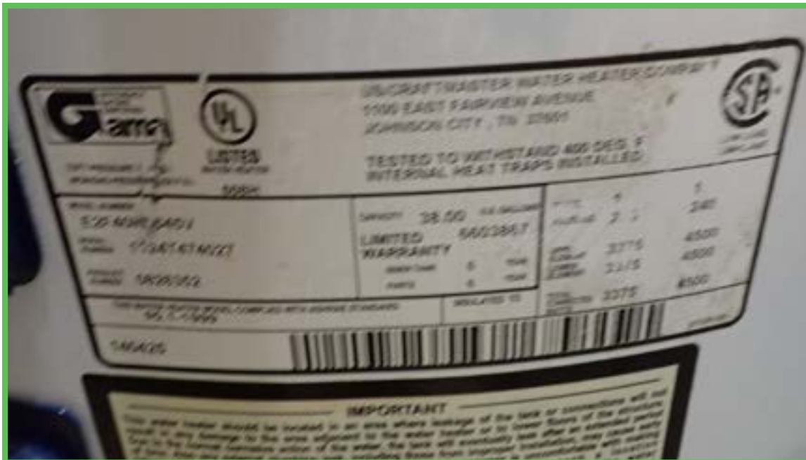
Water Heater Data Plate
