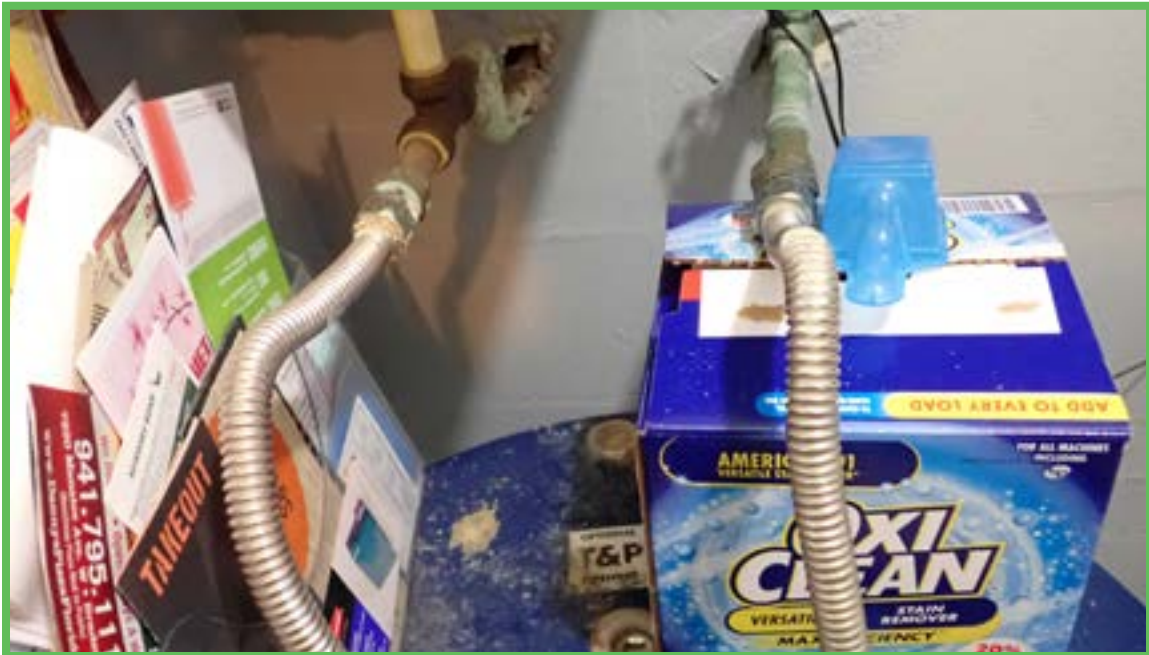
Hot Water Heater Plumbing Connections
