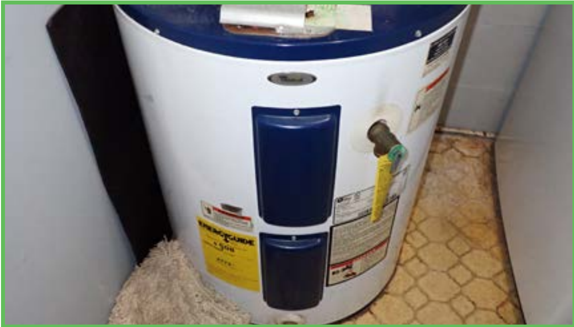
Hot Water Heater
