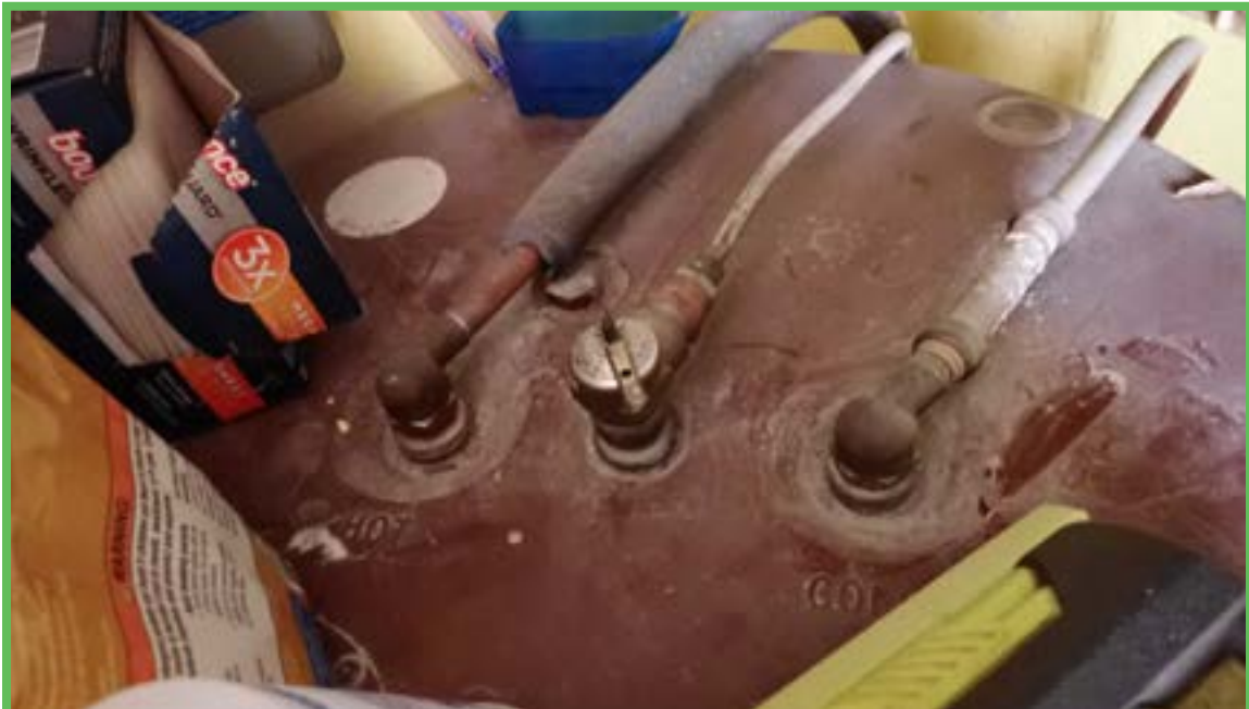
Hot Water Heater Plumbing Connections
