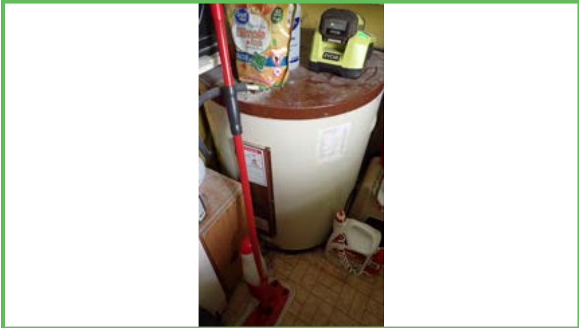
Hot Water Heater
