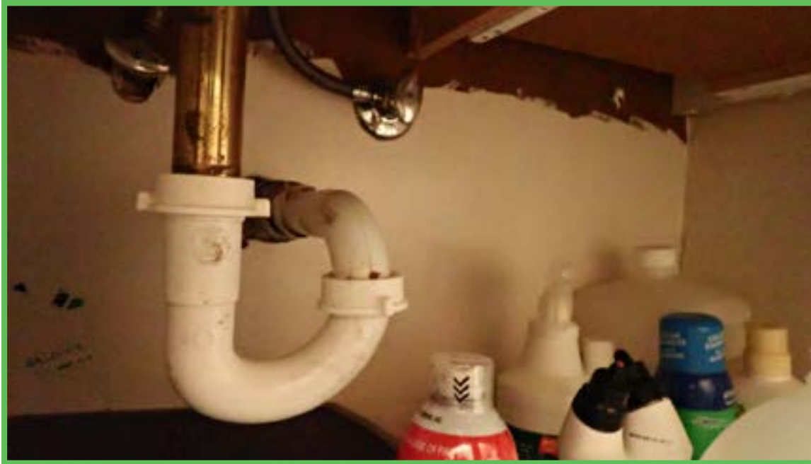
Under Sink1 Bath 1
