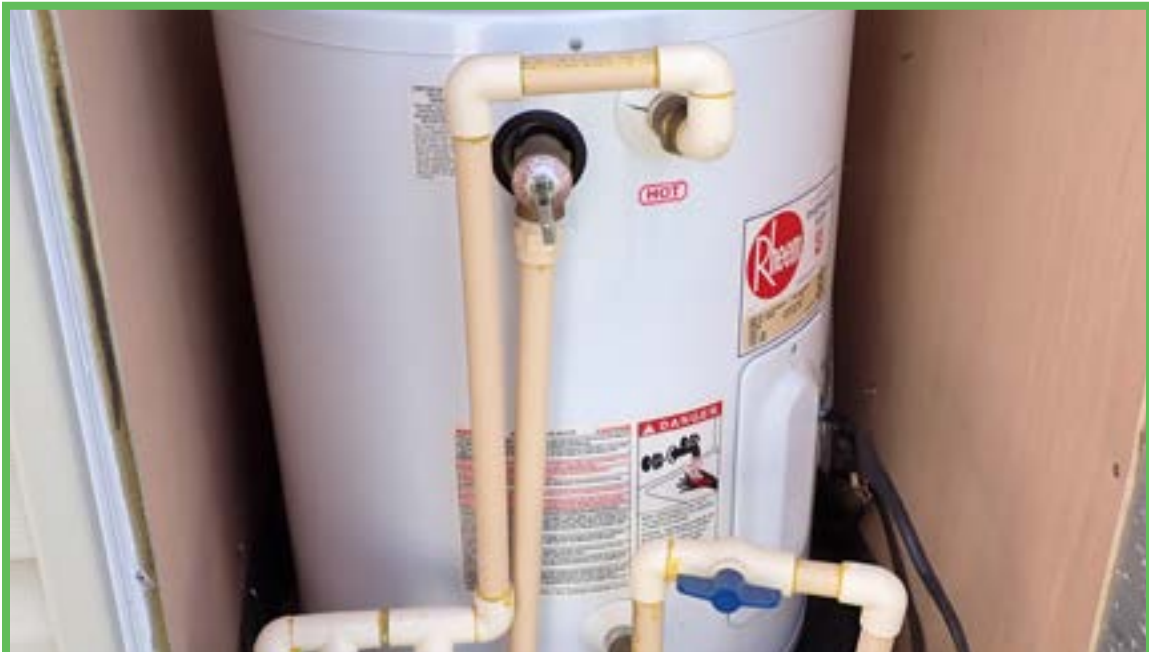
Hot Water Heater Plumbing Connections
