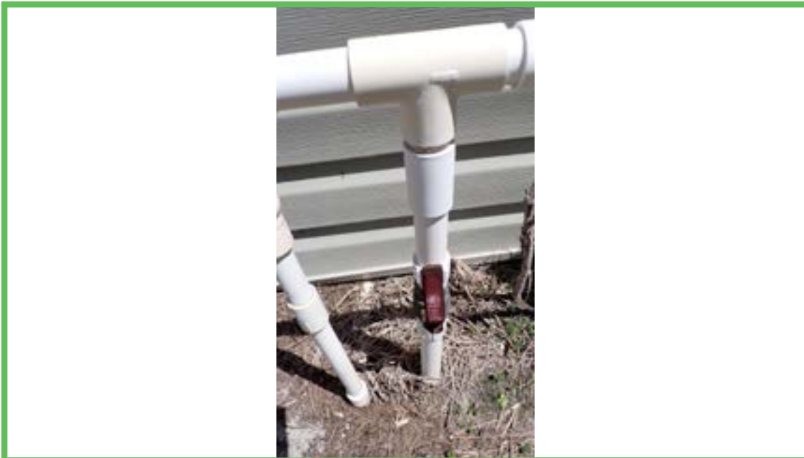
Main Water valve
