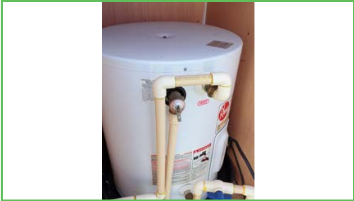
Hot Water Heater
