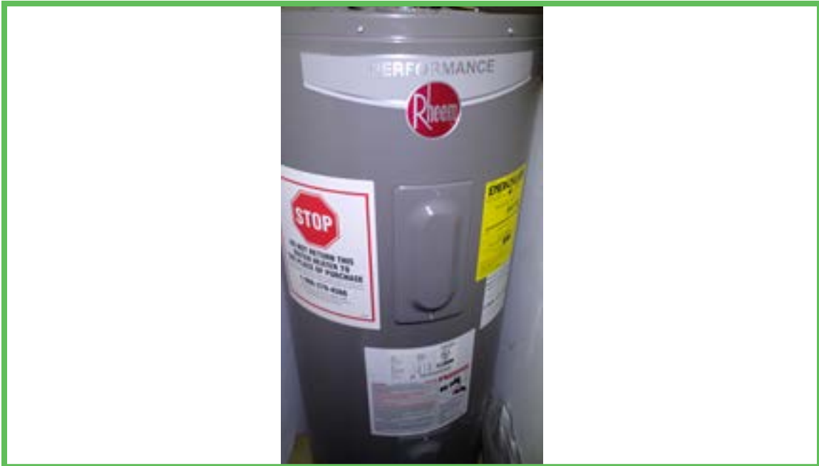
Hot Water Heater
