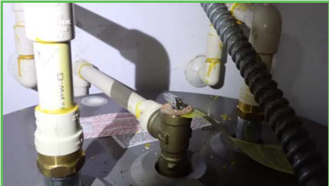
Hot Water Heater Plumbing Connections
