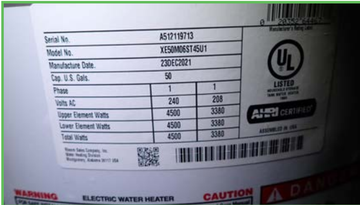
Water Heater Data Plate
