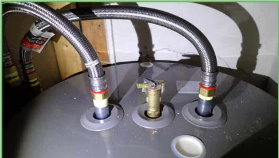
Hot Water Heater Plumbing Connections
