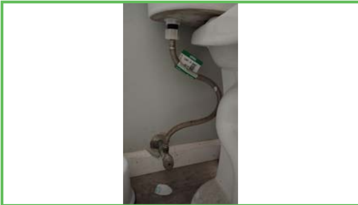
Bath 2 Toilet Valve
