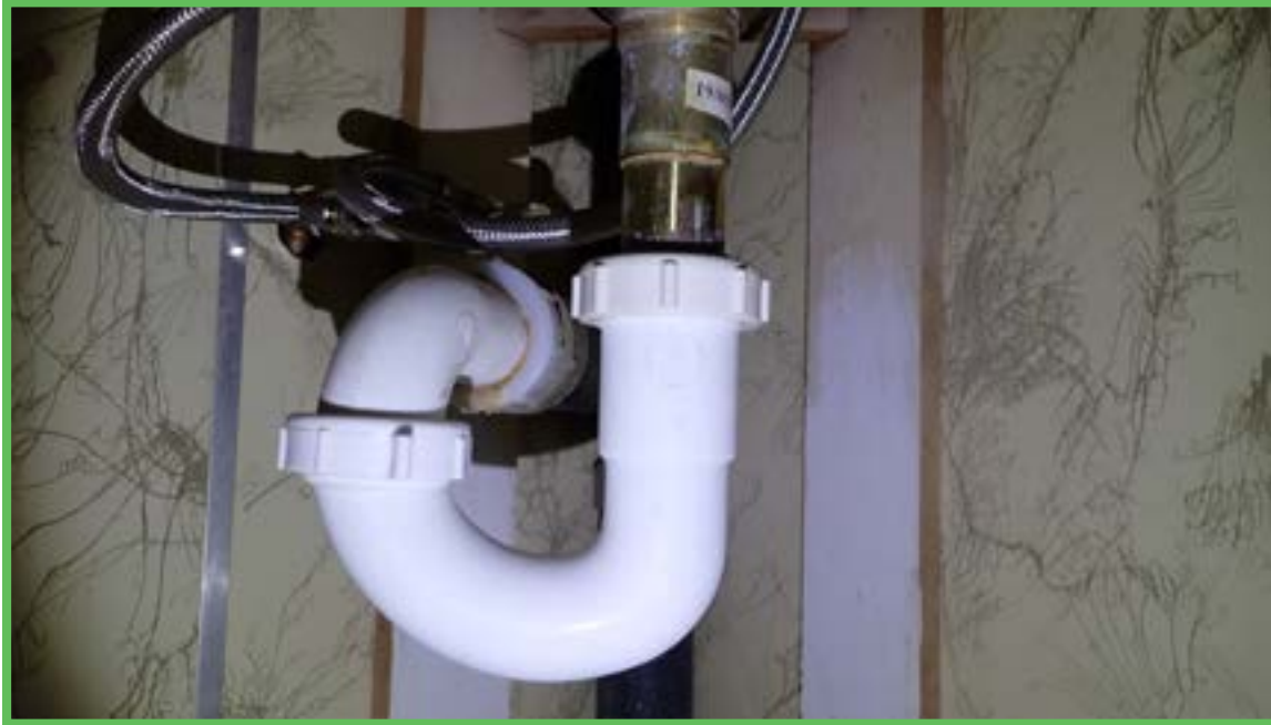
Under Sink1 Bath 1
