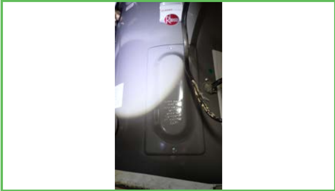
Hot Water Heater
