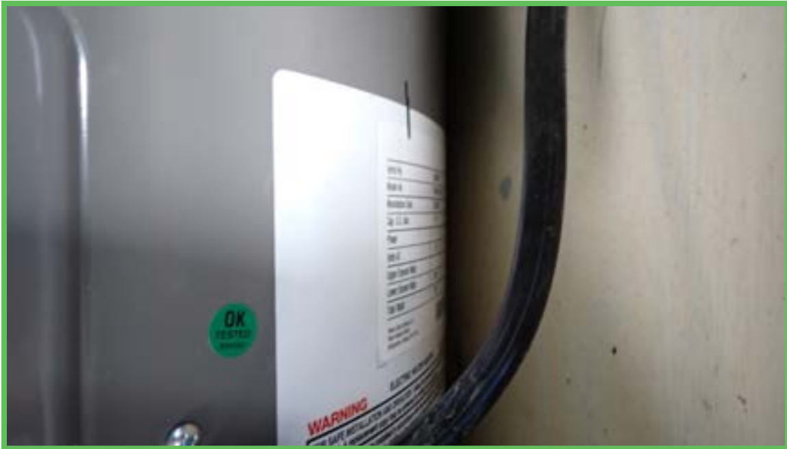
Water Heater Data Plate
