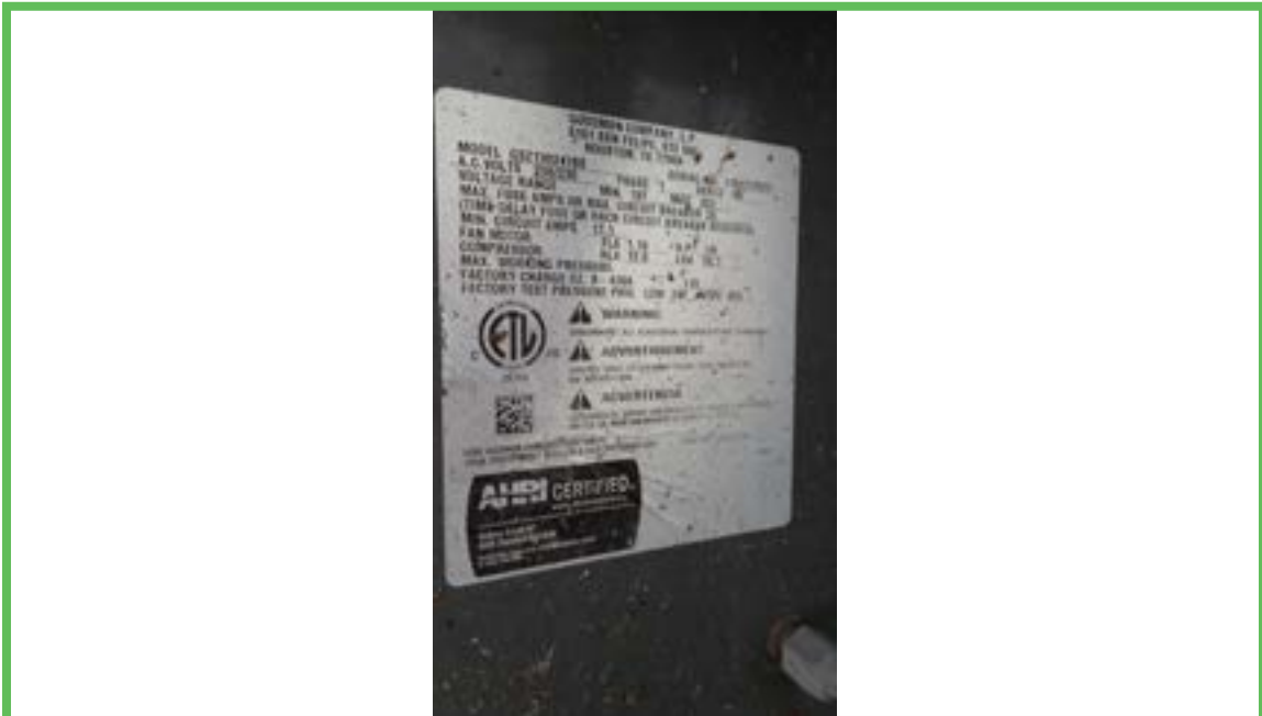
HVAC Condenser Data Plate
