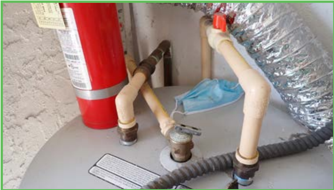
Hot Water Heater Plumbing Connections
