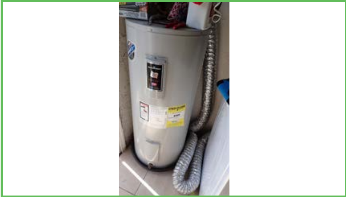
Hot Water Heater
