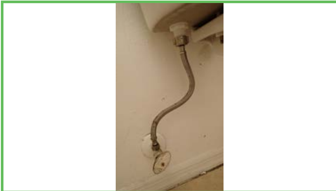
Bath 1 Toilet Valve
