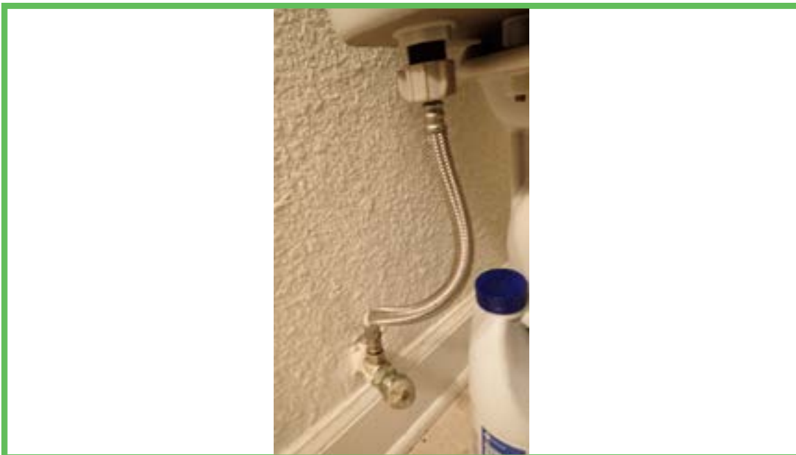
Bath 1 Toilet Valve
