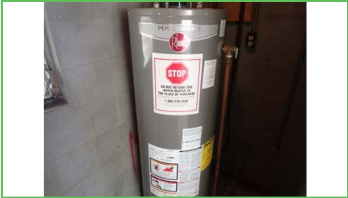
Hot Water Heater
