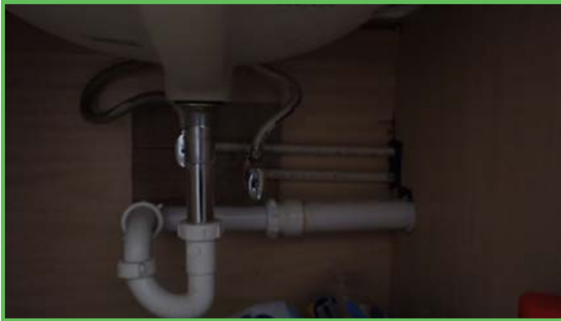
Under Sink1 Bath 2
