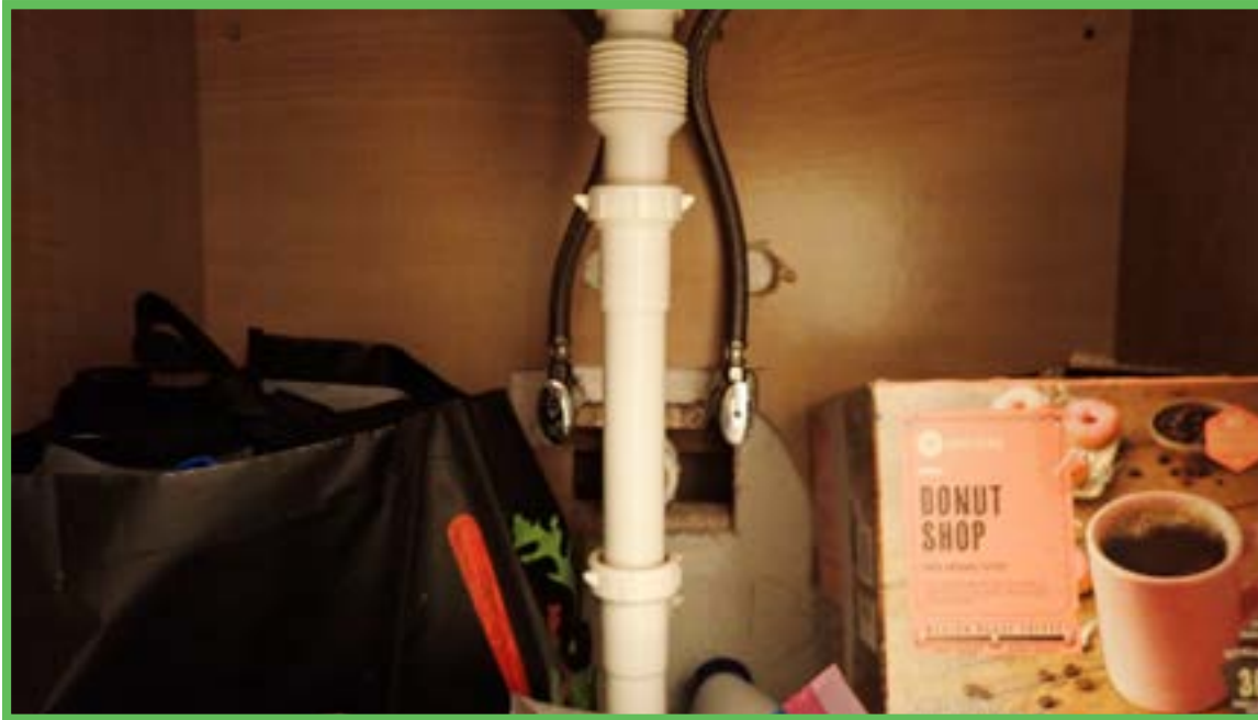
Under Sink1 Bath 1
