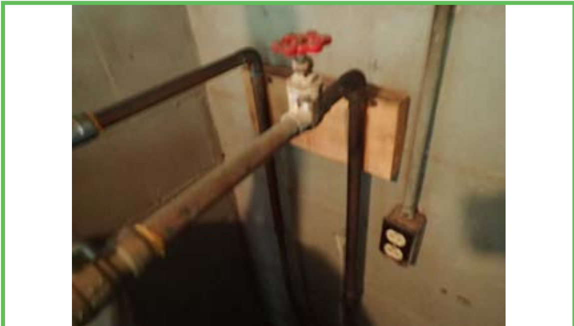
Hot Water Heater Plumbing Connections
