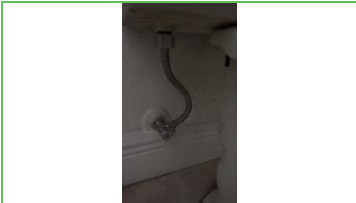
Bath 2 Toilet Valve
