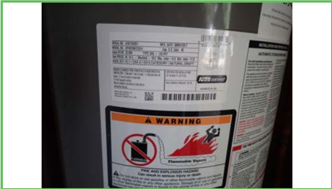
Water Heater Data Plate
