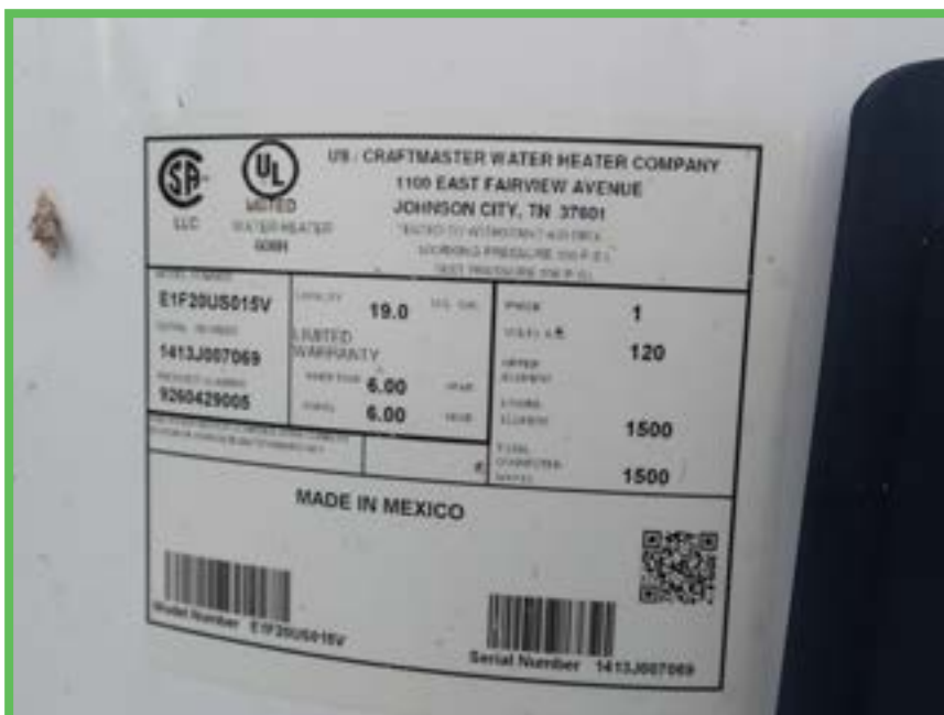
Water Heater Data Plate
