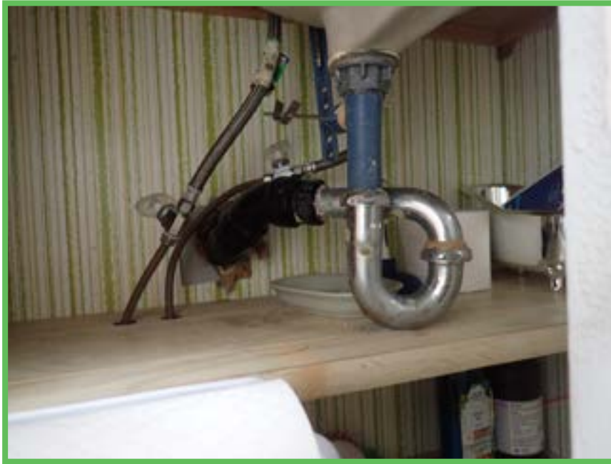
Under Sink1 Bath 1
