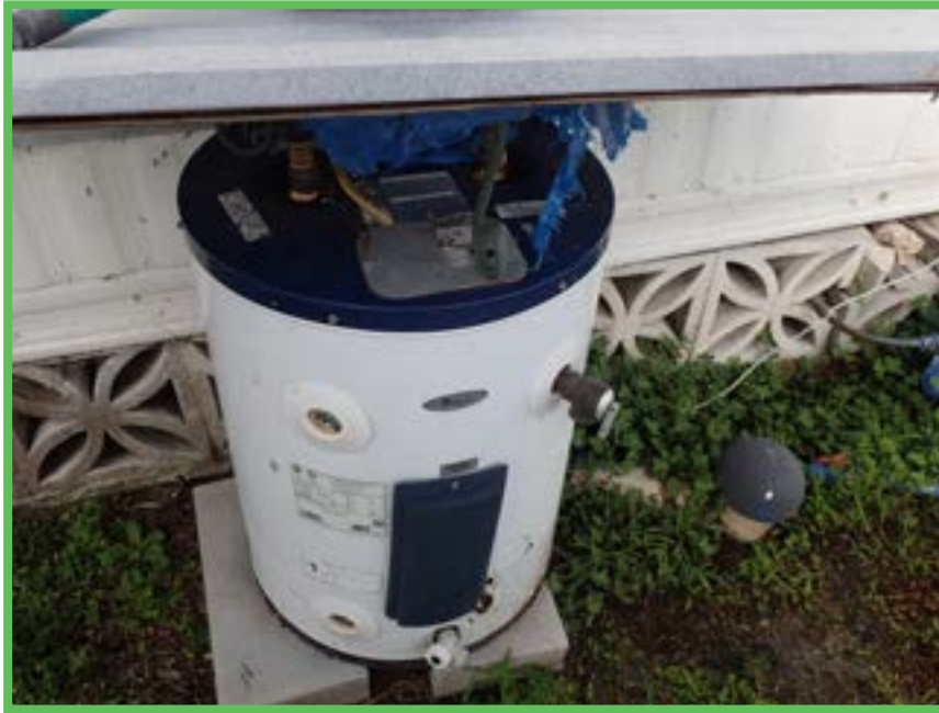
Hot Water Heater
