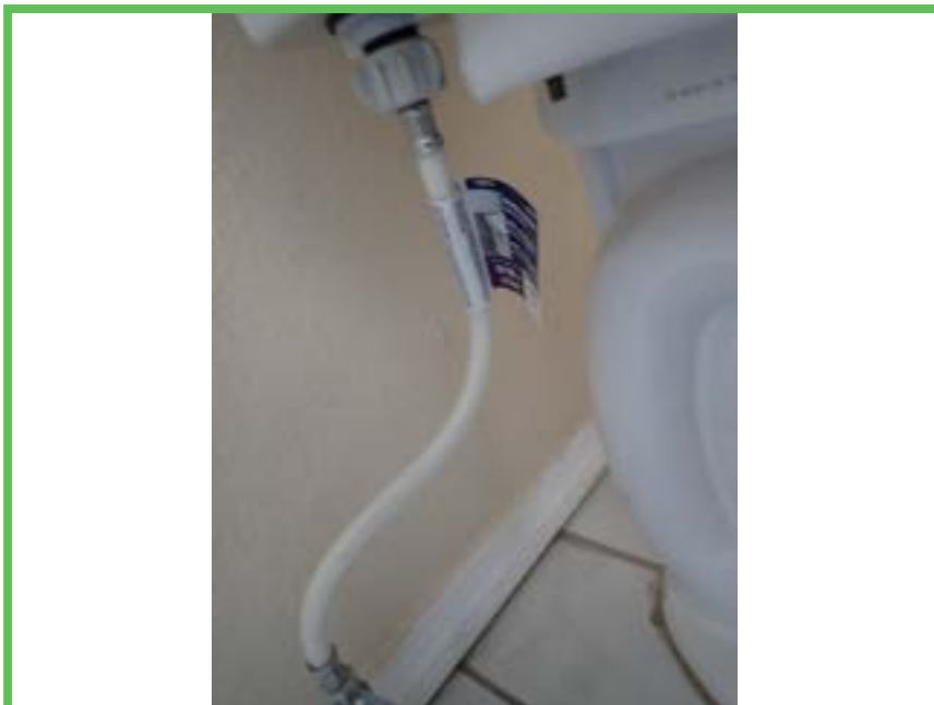
Bath 1 Toilet Valve
