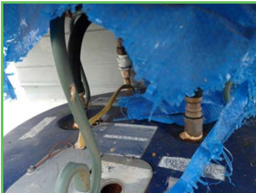
Hot Water Heater Plumbing Connections
