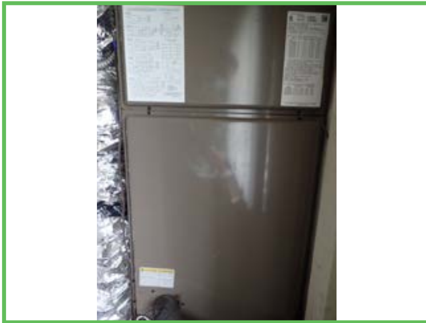
HVAC Air Handler
