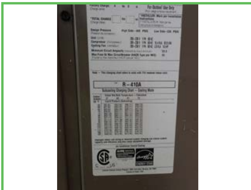
HVAC Condenser Data Plate
