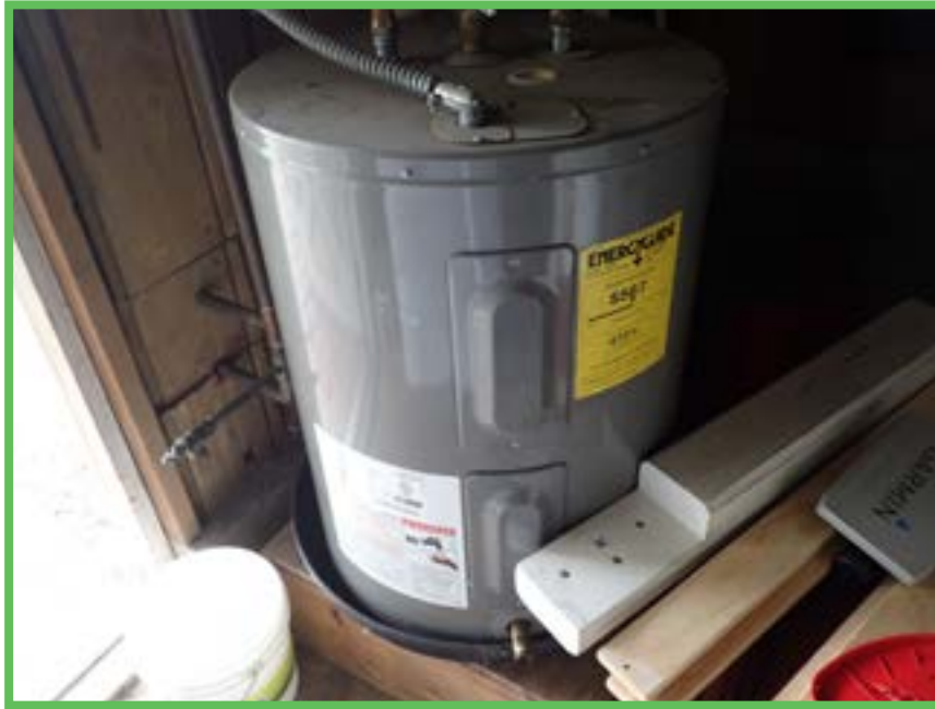
Hot Water Heater
