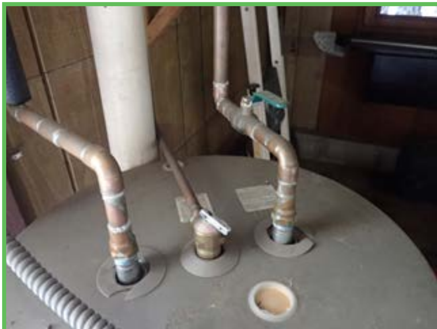
Hot Water Heater Plumbing Connections
