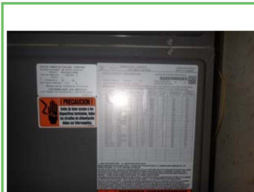
HVAC Air Handler Data Plate
