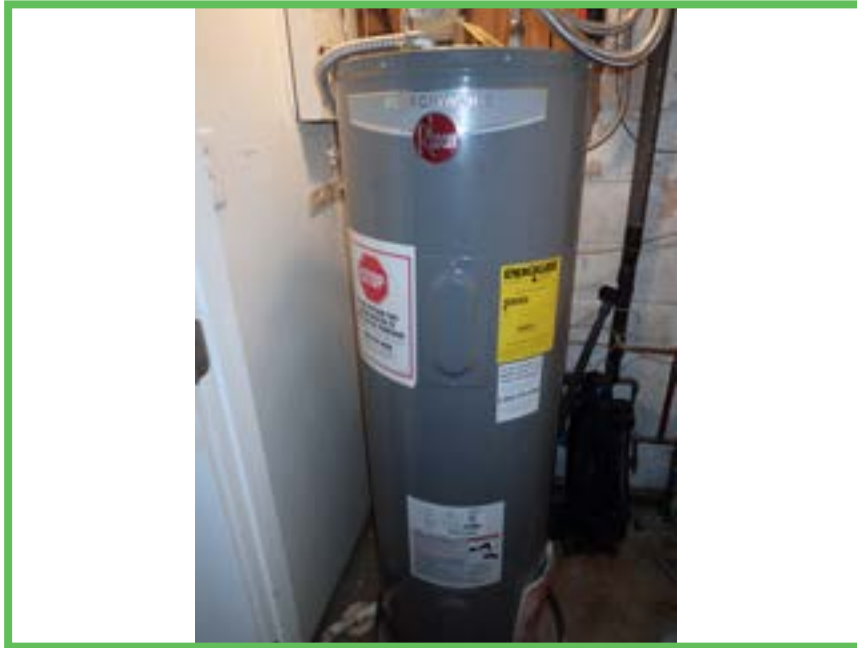
Hot Water Heater
