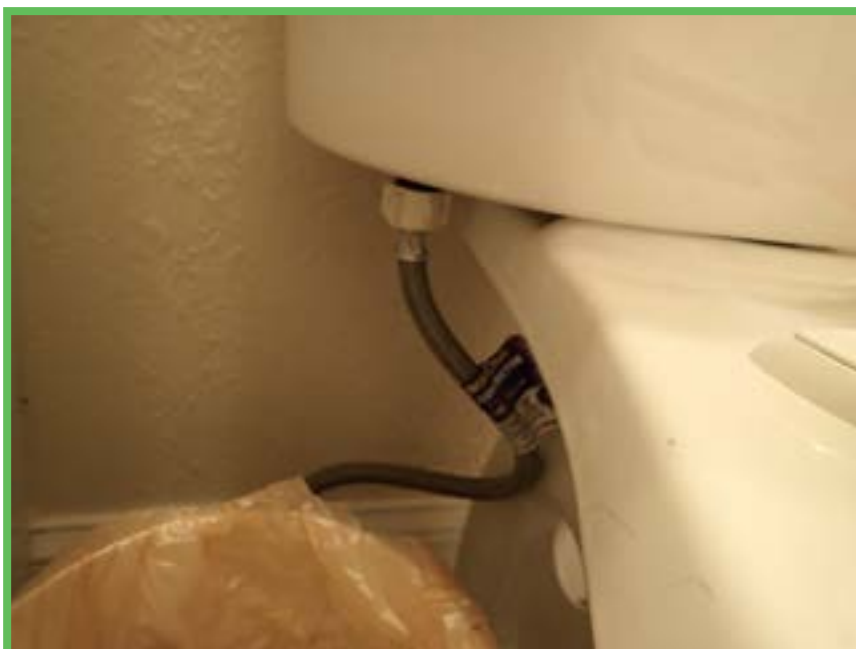
Guest Bath Toilet Valve
