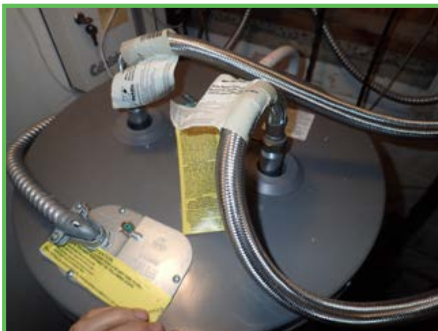
Hot Water Heater Plumbing Connections
