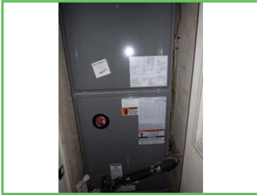
HVAC Air Handler
