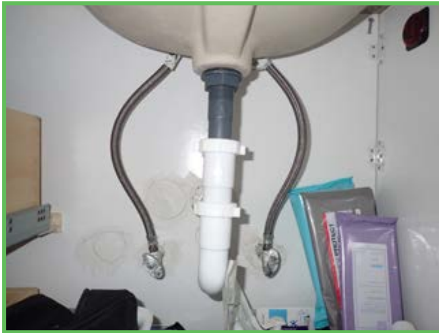
Under Sink Master Bath
